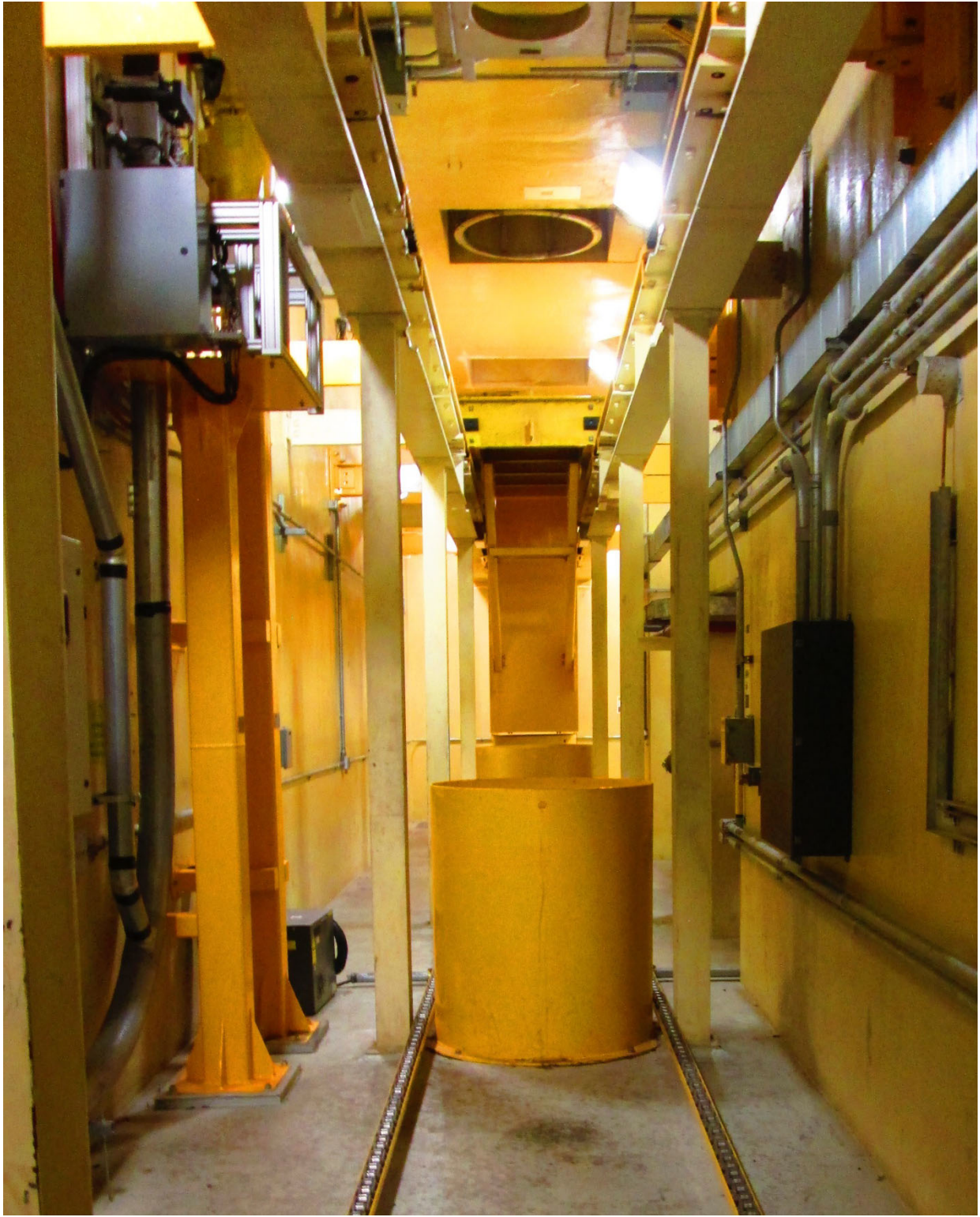
Figure B4-1044 Transfer Cell
