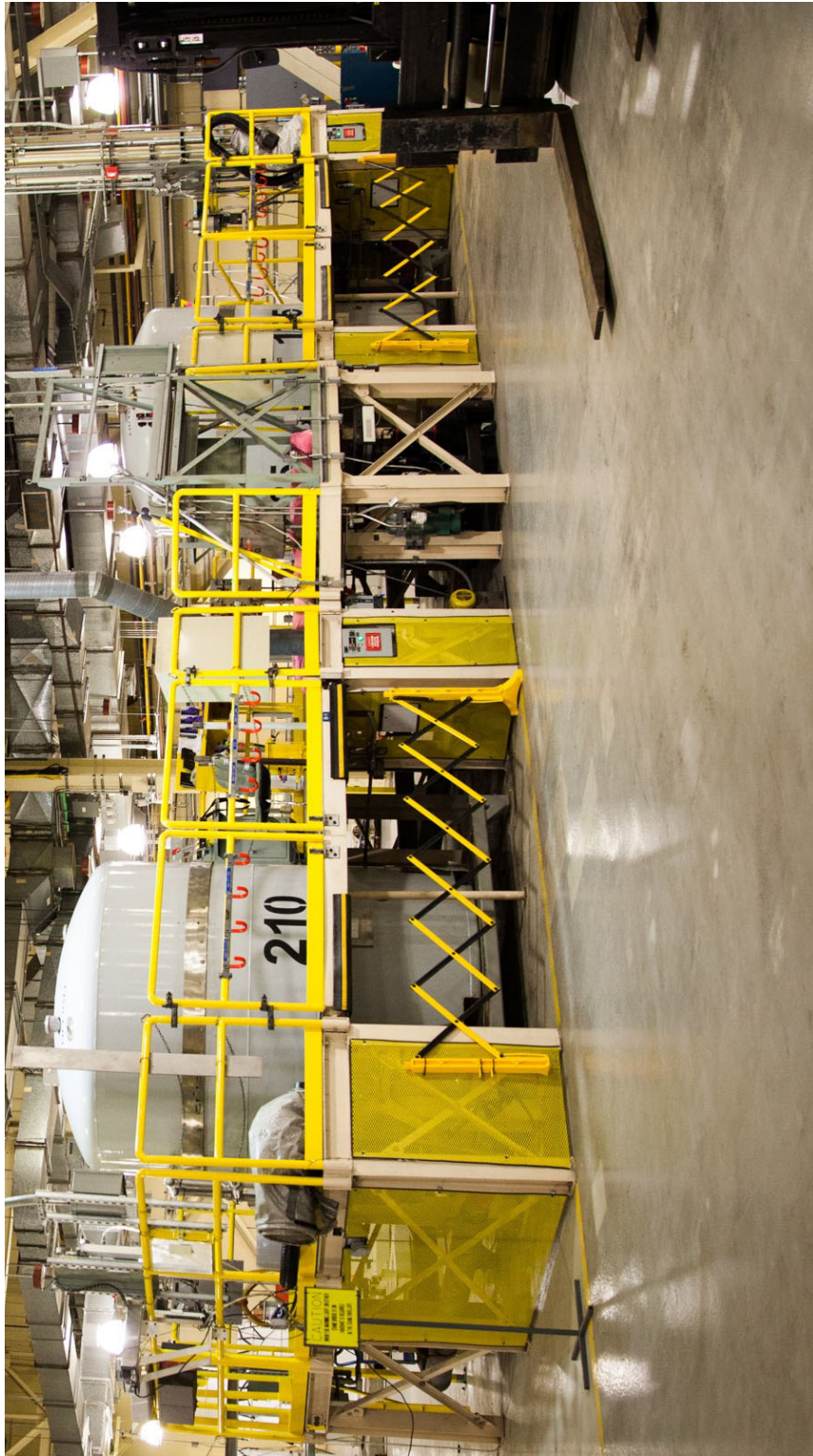
Figure B4-4 TRUDOCKs (East) in CH Bay of the Waste Handling Building
