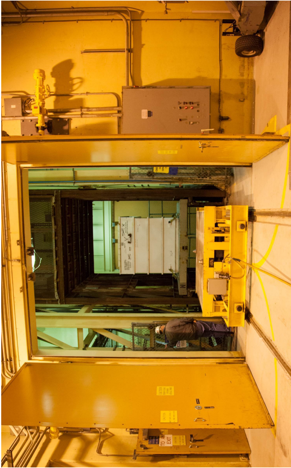
Figure B4-67 Waste Shaft Conveyance - Loading Facility Pallet with CH Waste, Waste Handling Building
