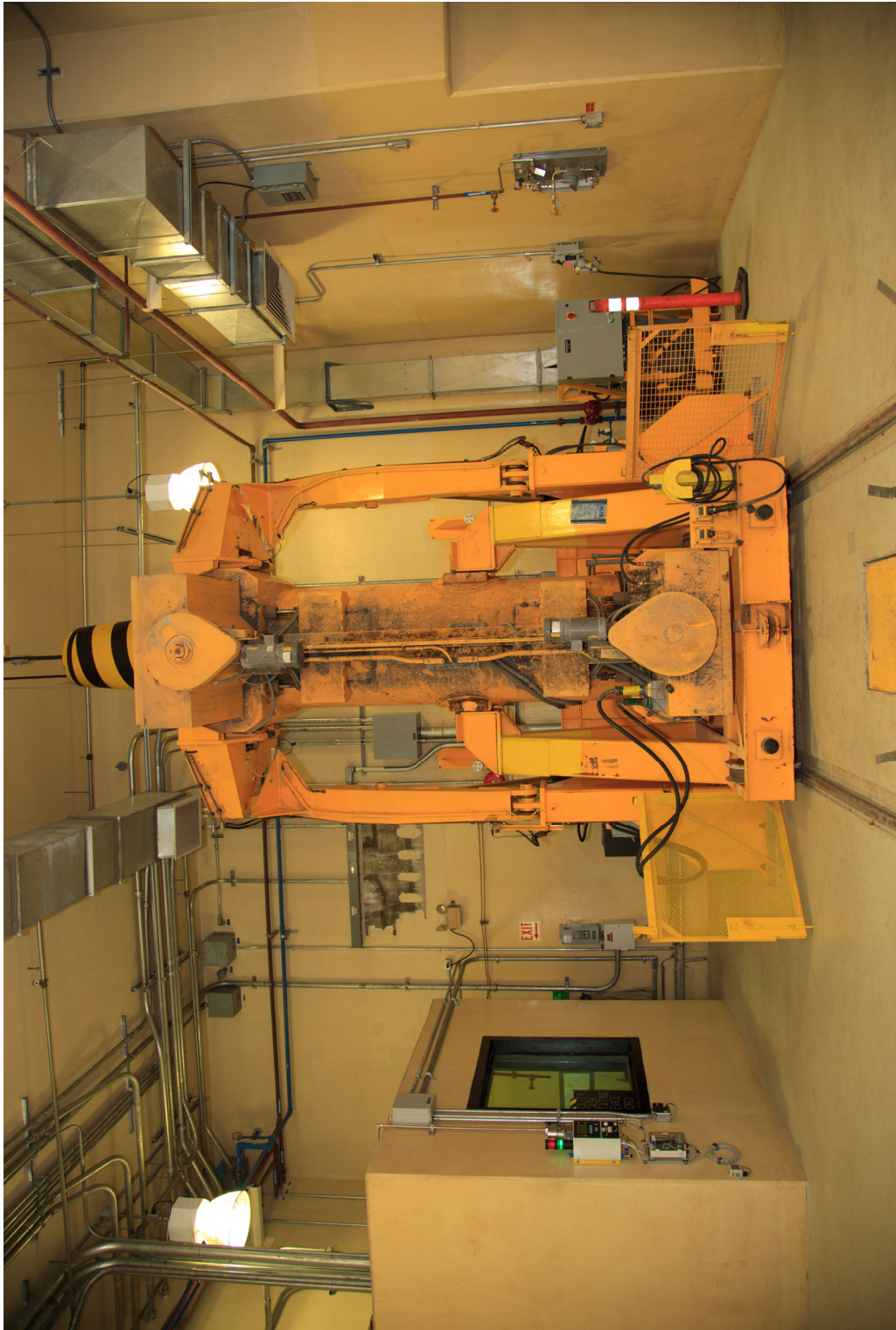
Figure B4-1142 Facility Cask Loading Room and Facility Cask Rotating Device
