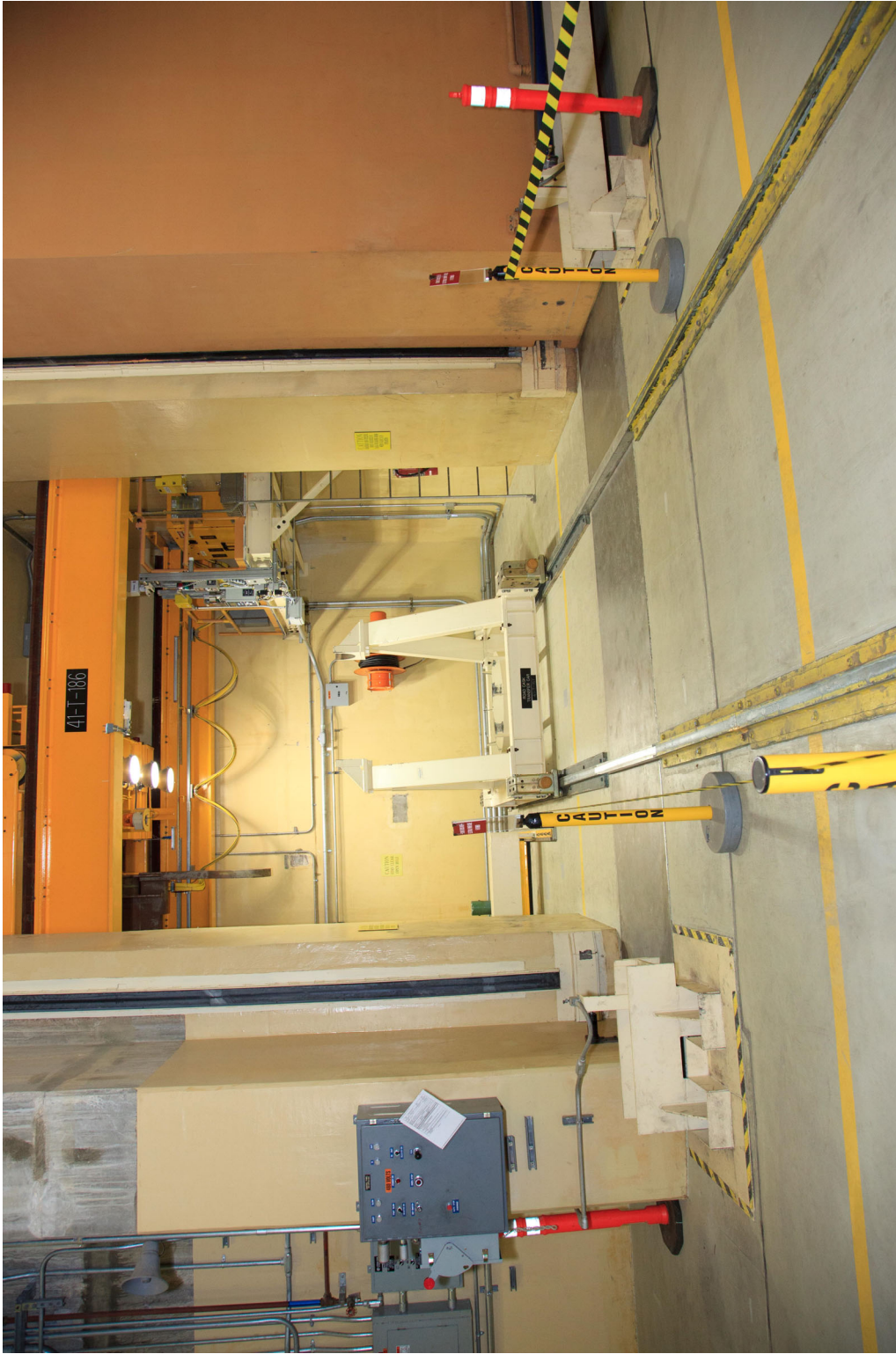
Figure B4-89 Cask Unloading Room and Bridge Crane
